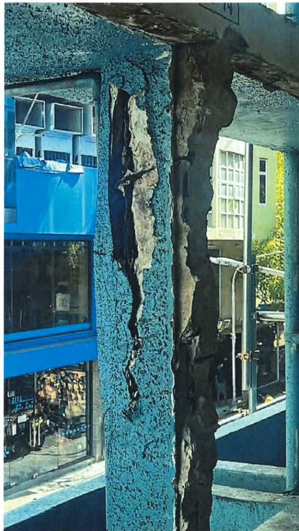
Figure 8 RC Column spalling damage, 1st floor
