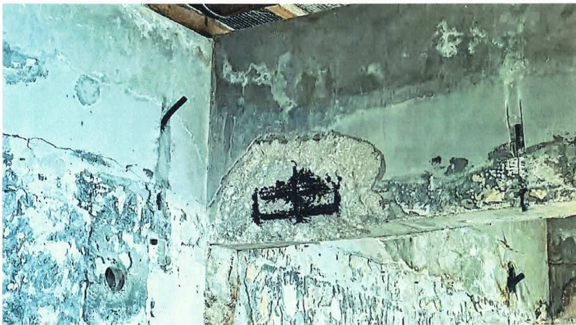
Figure 4 RC Beam, spalling damage, 2 nd floor
