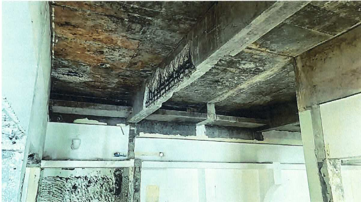
Figure 3 RC Beam showing extensive spalling, same as Figure 2 (opposing side).
