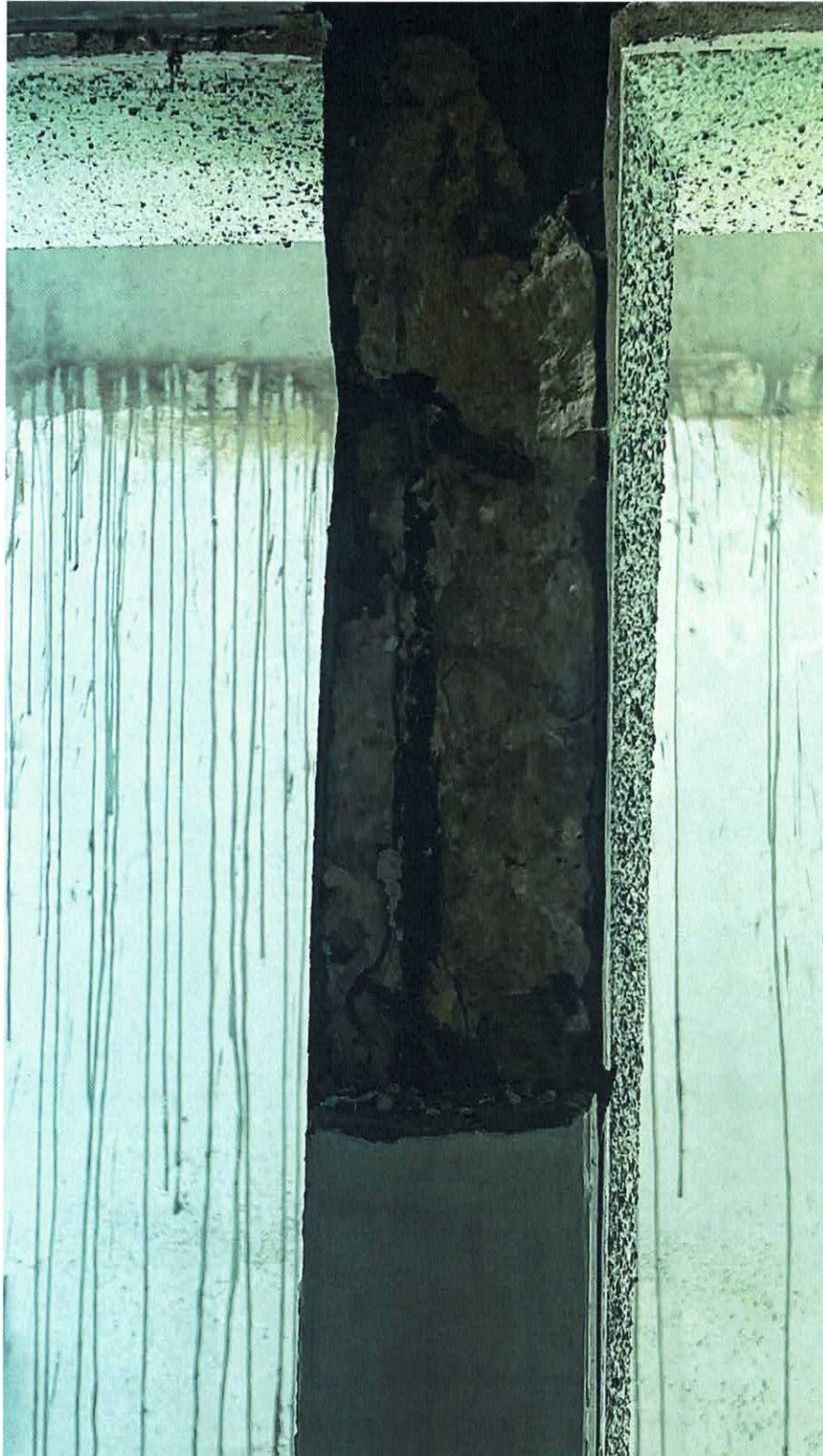
Figure 11 RC Column spalling damage
