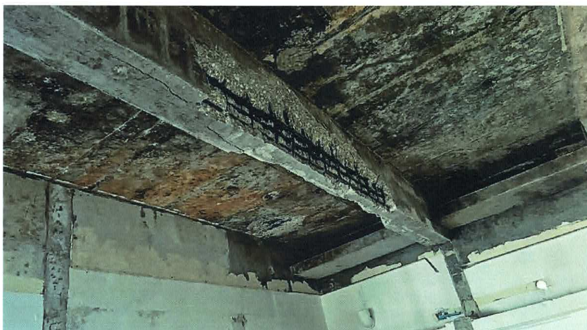
Figure 2 RC Beam with spalling damage, extensive up to 1.5m in length on long axis of beam, ground floor
