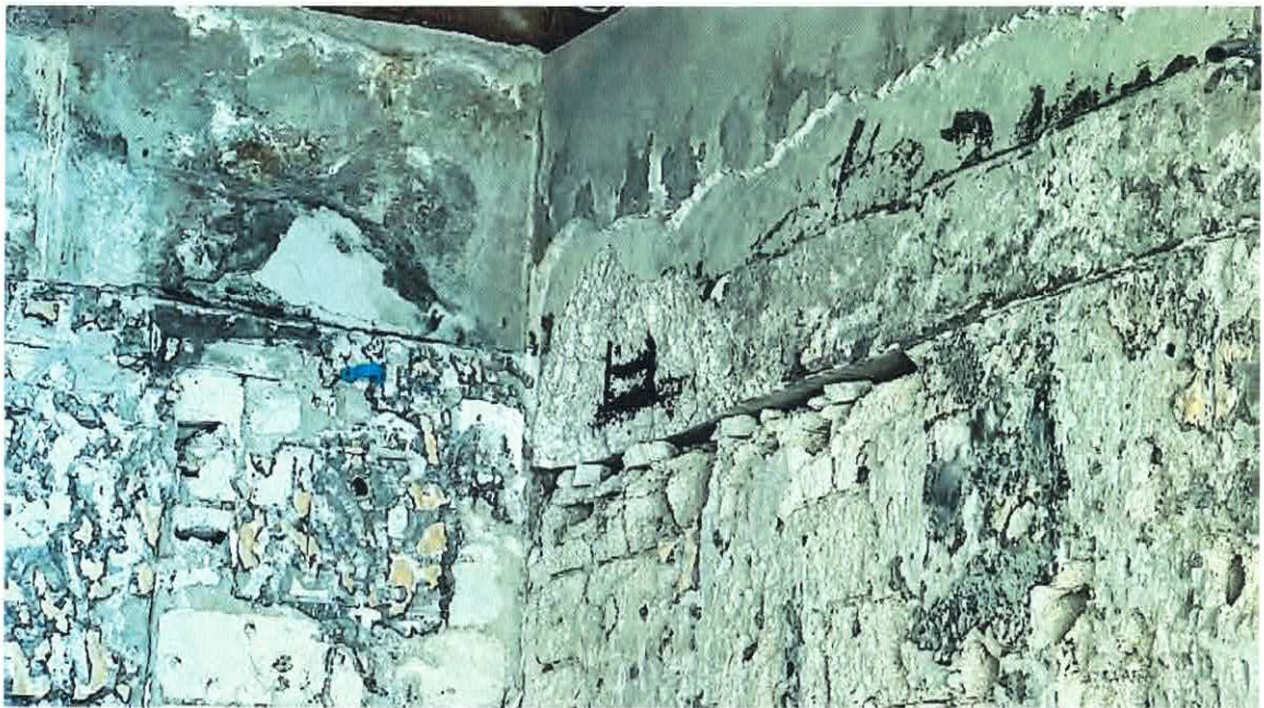
Figure 6 RC Beam spalling damage, 2nd floor
