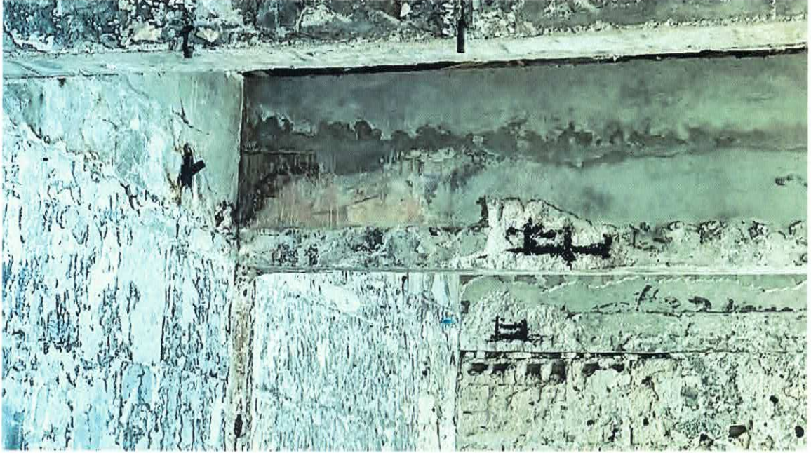
Figure 5 RC Beam spalling damages, 2nd floor
