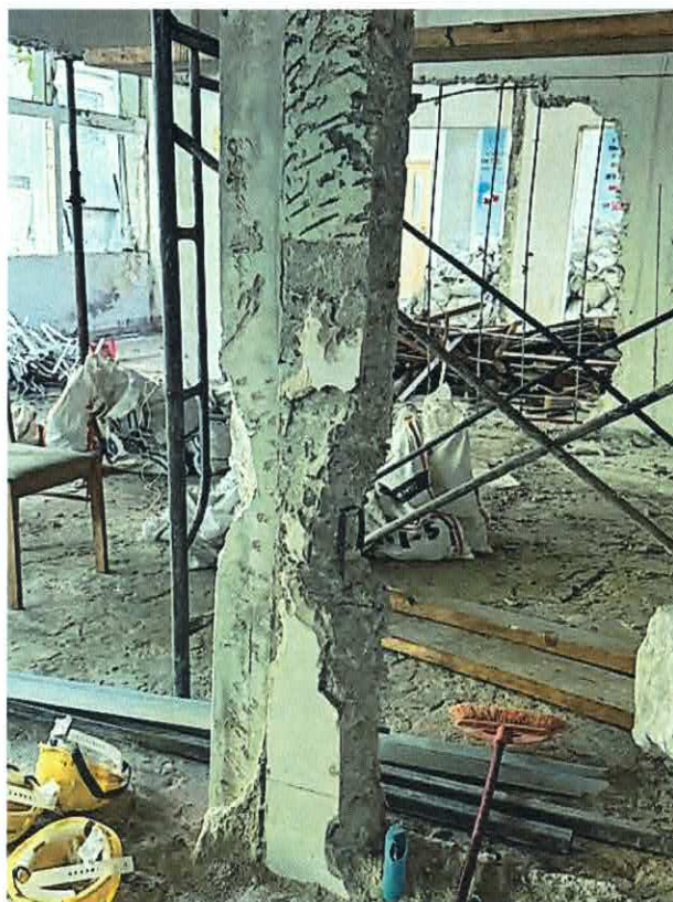
Figure 1. RC Column with spalling.
