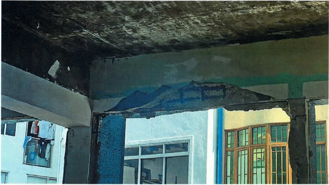
Figure 12 RC Beam, spalling damage, ground floor
