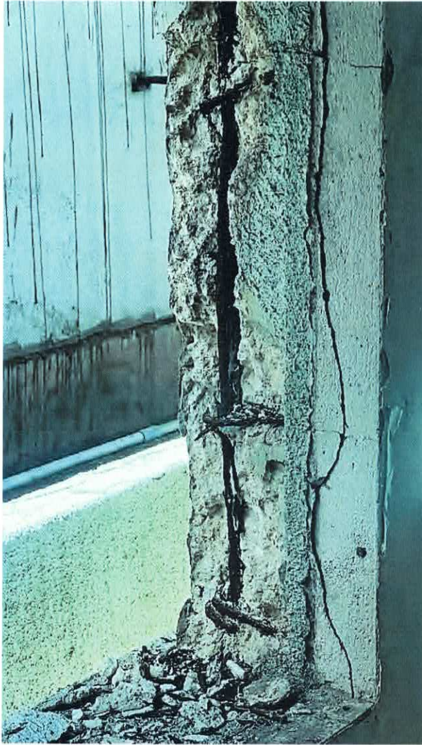
Figure 9 RC Column Spalling damage, ground floor.
